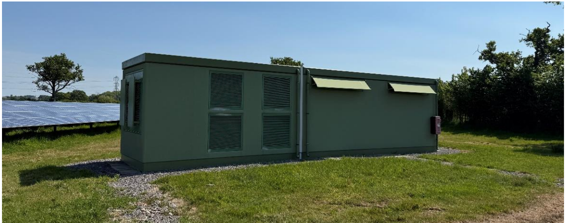
Insert 4-5 Sub-distribution Switch Room
