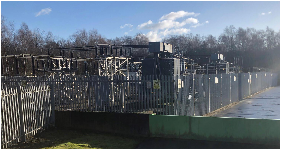
Insert 4-9 Typical 132kV substation compound
