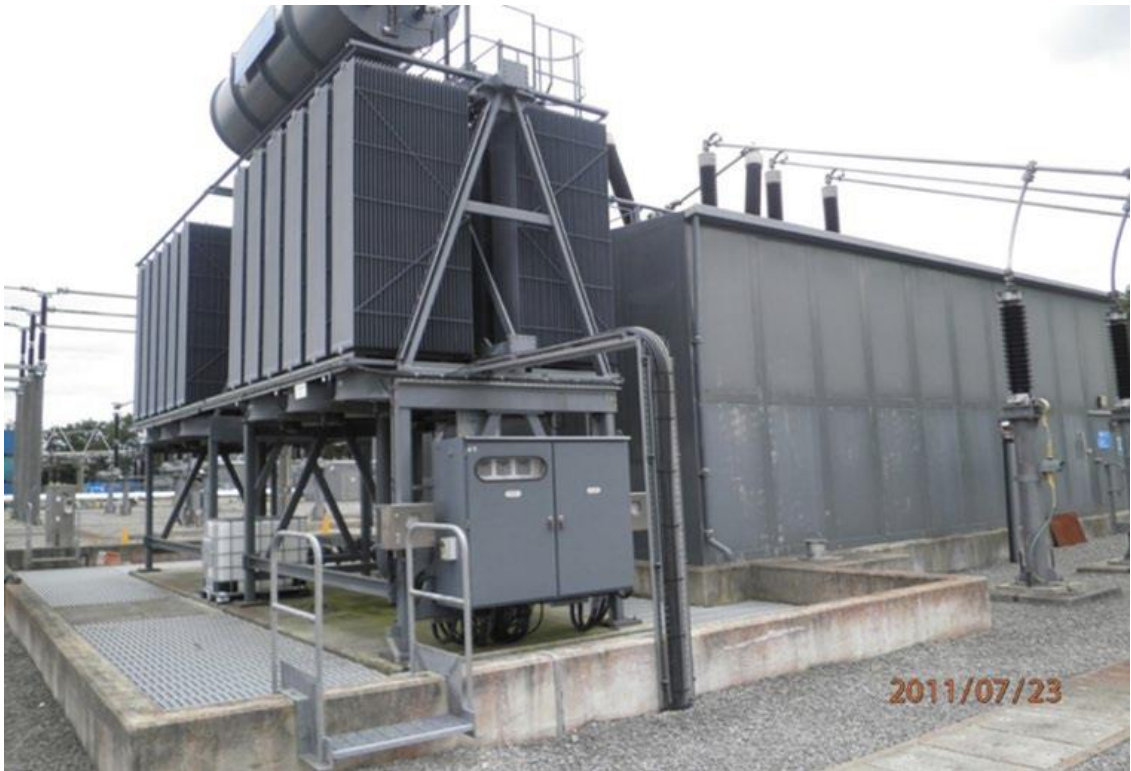
Insert 4-8 Typical (large 400kV) power transformer
