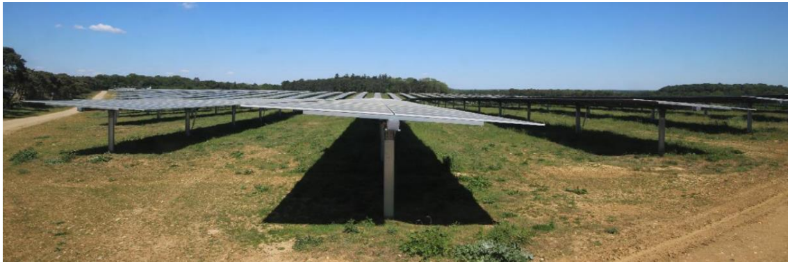
Insert 4-2 Typical Tracker Solar Panels in a Near Flat Orientation
